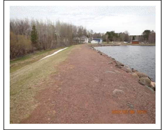
42. Gile Dam Canoe Portage – East side of dam, riprap shoreline of flowage
