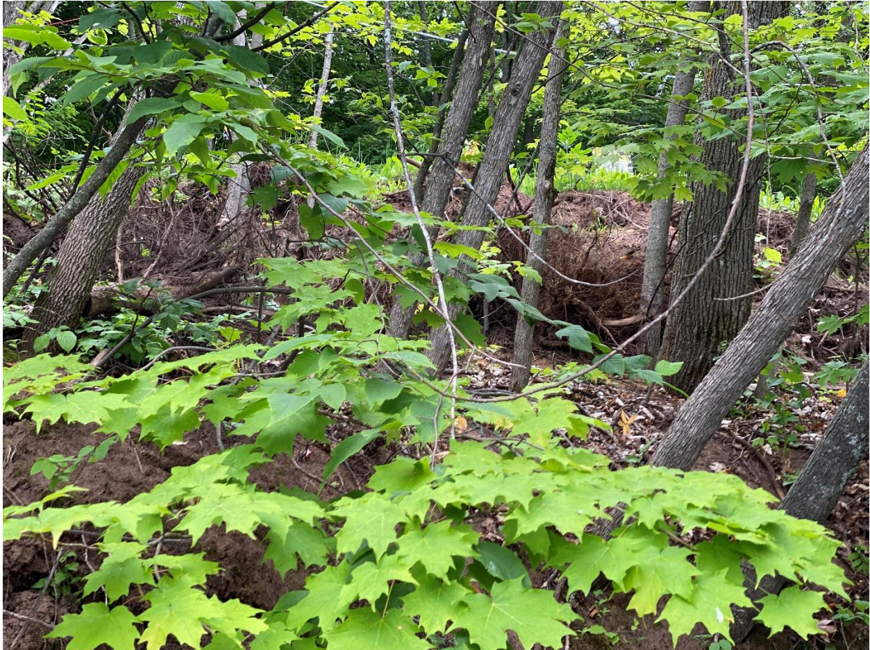
FIGURE 4f. SITE #5 GILE FLOWAGE (July 17, 2023). CLOSEUP PHOTOGRAPH OF BANK INSTABILITY
