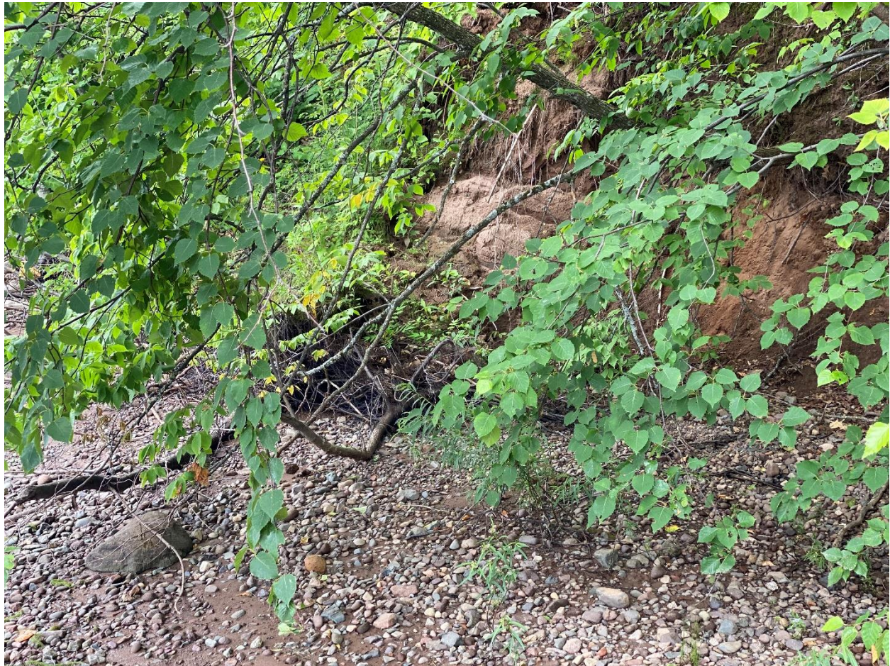
FIGURE 4h. SITE #5 GILE FLOWAGE (July 17, 2023). CLOSEUP PHOTOGRAPH OF BANK INSTABILITY
