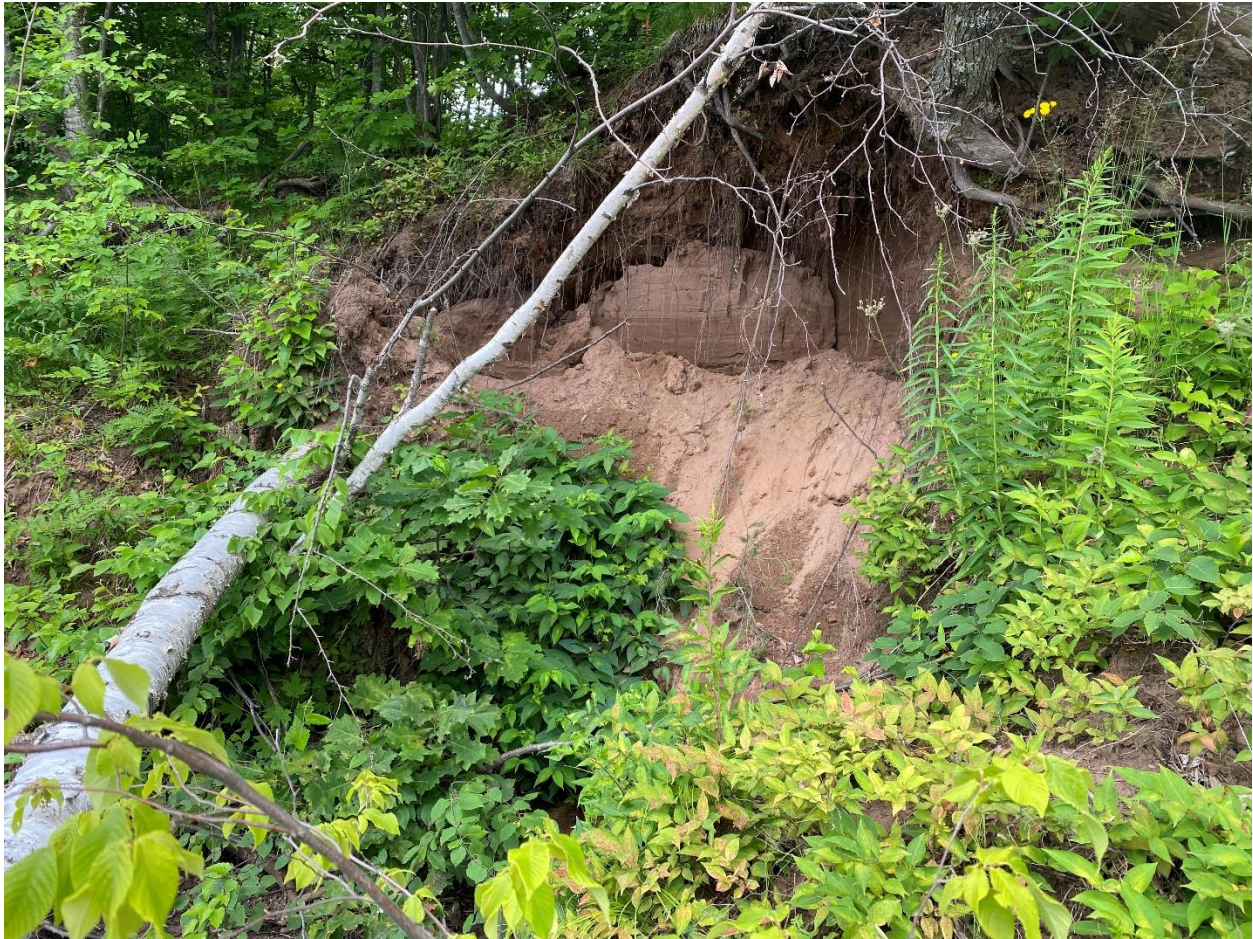
FIGURE 4c. SITE #5 GILE FLOWAGE (July 17, 2023). CLOSEUP PHOTOGRAPH OF BANK INSTABILITY
