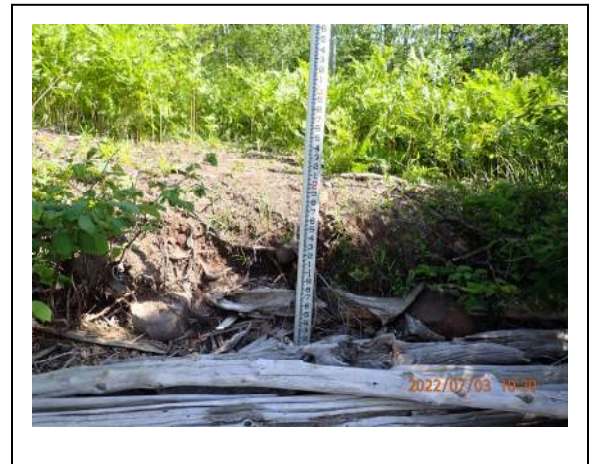
96. Island #20 – Bank erosion
