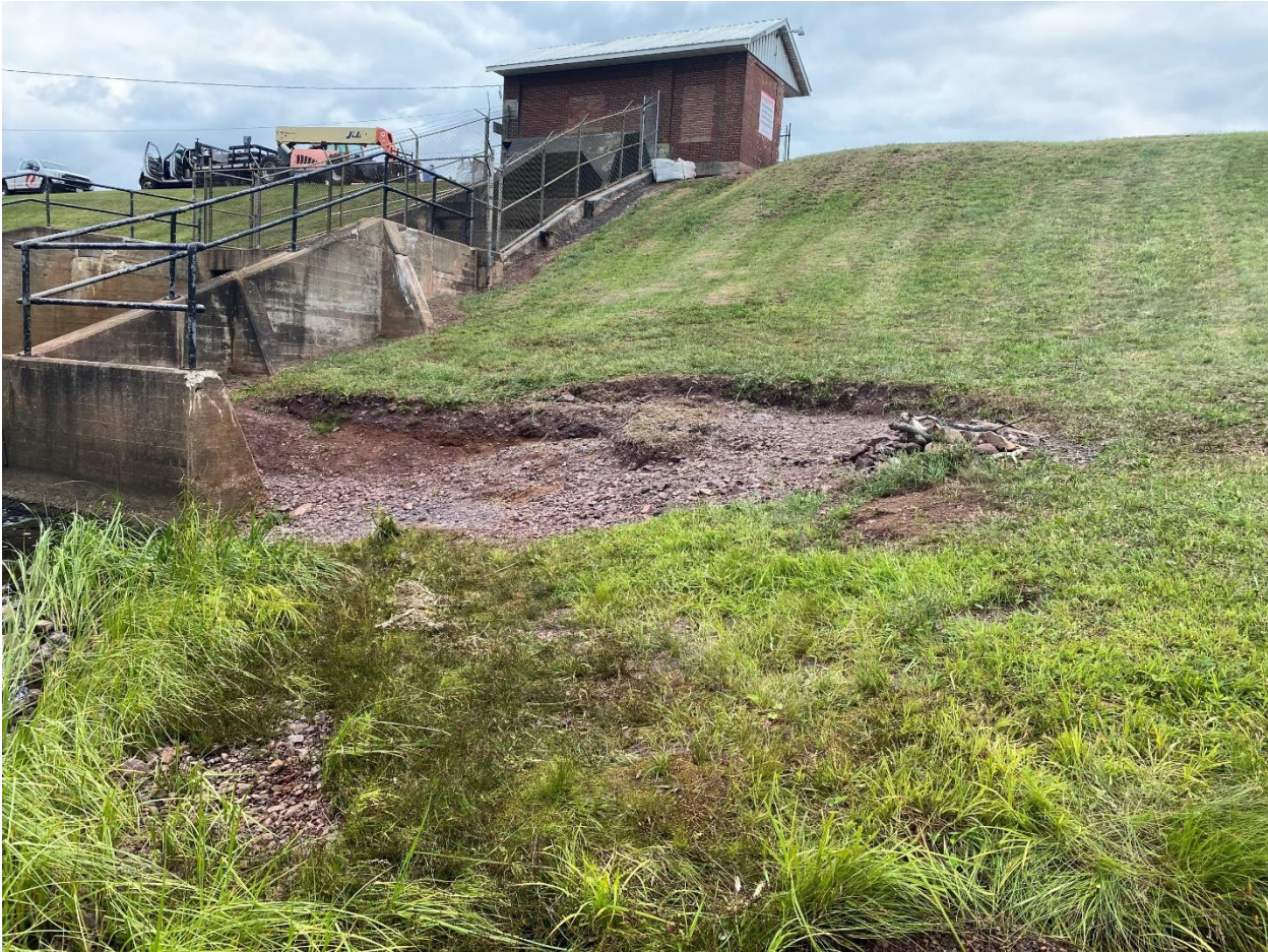
FIGURE 3. AREA OF INTEREST ON THE LEFT EMBANKMENT (WEST WINGWALL) AT THE TOW OF THE EMBANKMENT (July 17, 2023).
