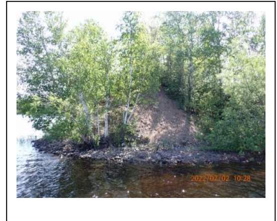
42. Island #9 - Bank erosion
