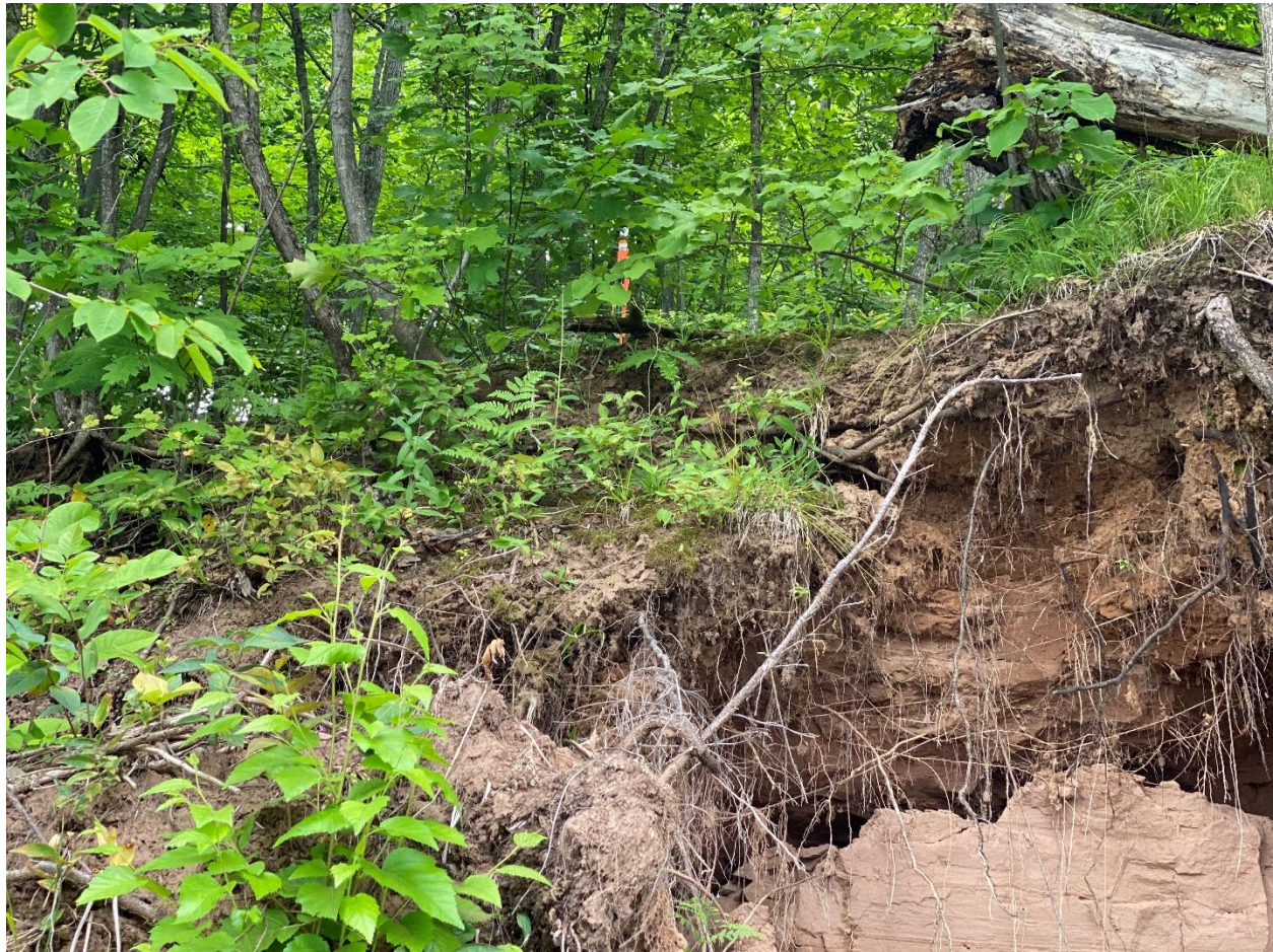
FIGURE 4c. SITE #5 GILE FLOWAGE (July 17, 2023). CLOSEUP PHOTOGRAPH OF BANK INSTABILITY (SEE SURVEY MARKER AT TOP OF PHOTOGRAPH NEAR EXCAVATION SITE)
