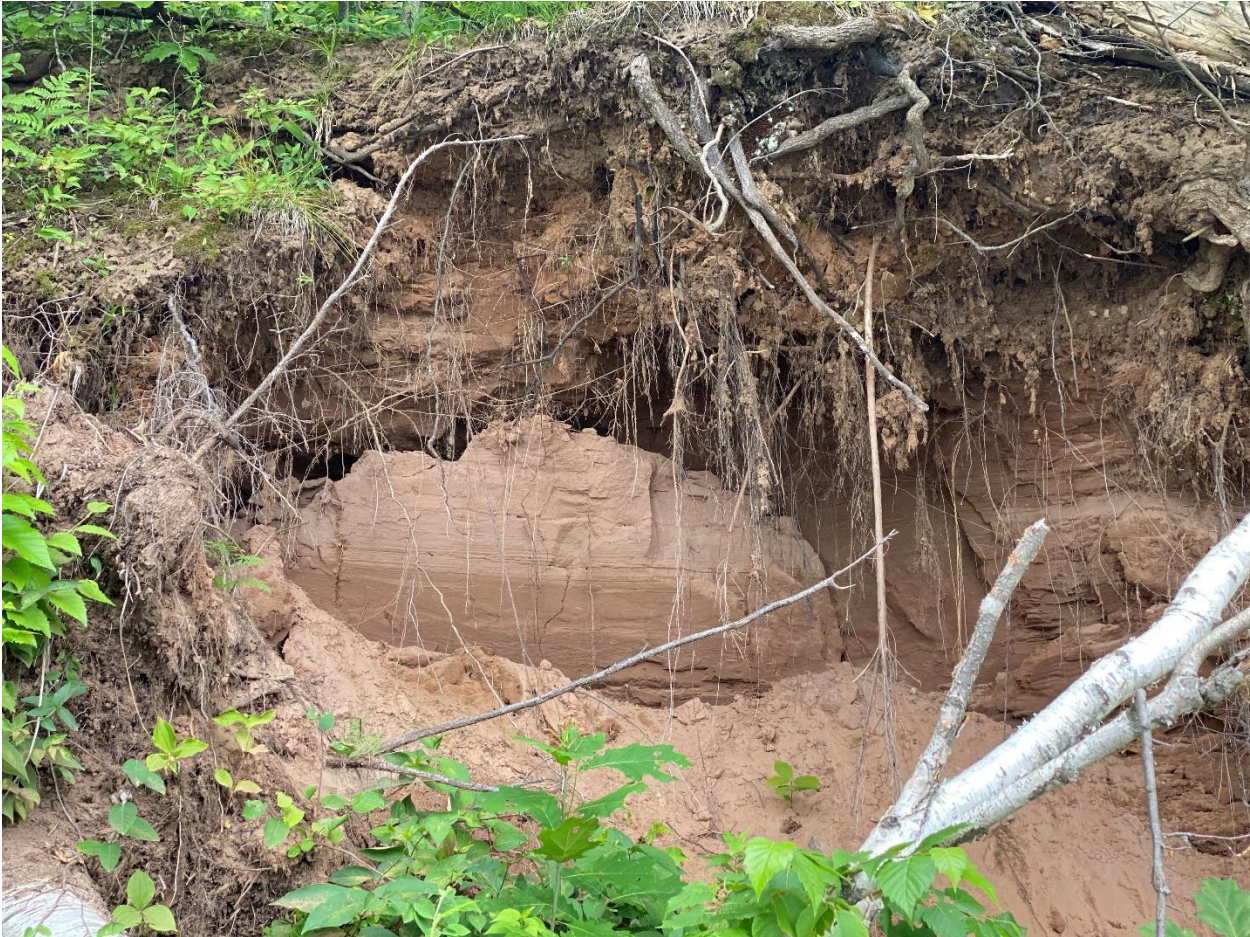
FIGURE 4e. SITE #5 GILE FLOWAGE (July 17, 2023). CLOSEUP PHOTOGRAPH OF BANK INSTABILITY
